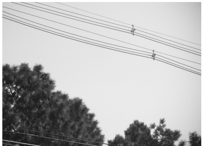
Bundle cables provide a method for reducing the space needed for overhead lines and therefore the amount of pruning necessary to pass lines through the top of a tree.
