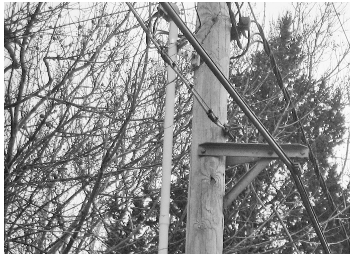
Alley arms can sometimes be used to route power lines to the outside of tree crowns, reducing the need for severe pruning.
